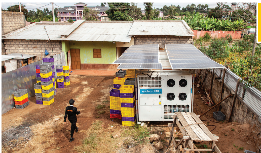
A solar-powered cold room facility for storing farm produce
